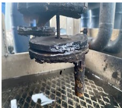
Figure 2 - Image of methane vent post casualty.
